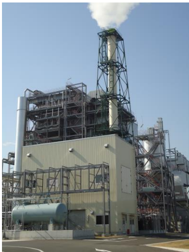
Biomass power plant in Kawasaki city, Kanagawa
